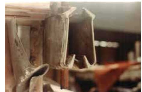
Figure 4. Deformed box beam failed connection.
