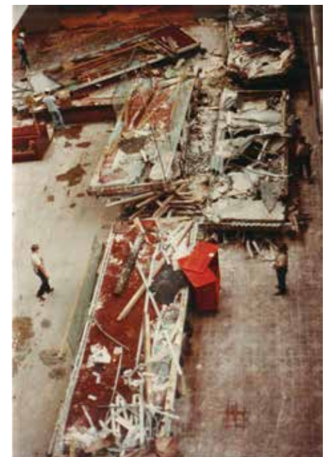
Figure 5. The collapsed second- and fourth-floor walkways on the floor of the atrium after the rescue operation.
