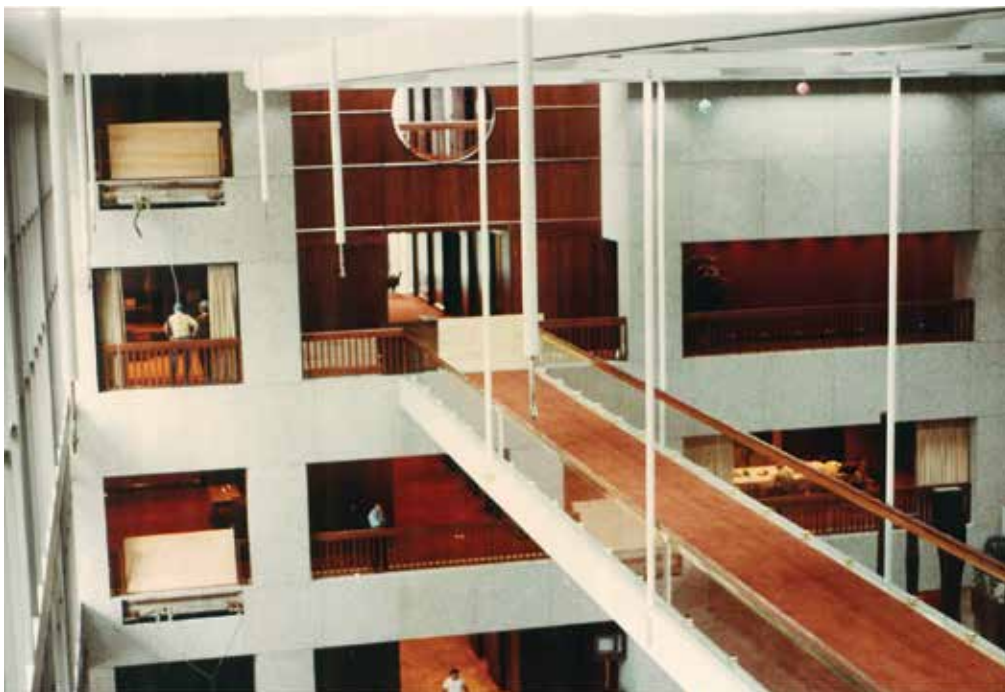
Figure 1. After the event; the fourth-floor hanger rods remain next to the intact third-floor walkway.
